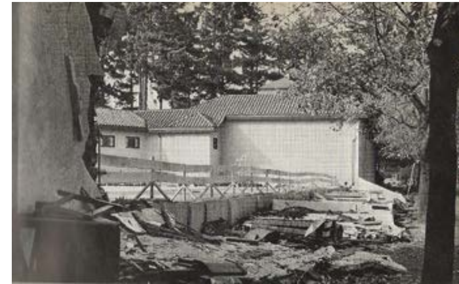
Peninsula Park swimming pool wall crashed to sidewalk after the Columbus Day storm of 1962
