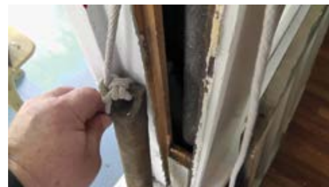
A homeowner accesses a double sash window’s counter weight, similar to the ones manufactured at Leach Brothers Iron Works
